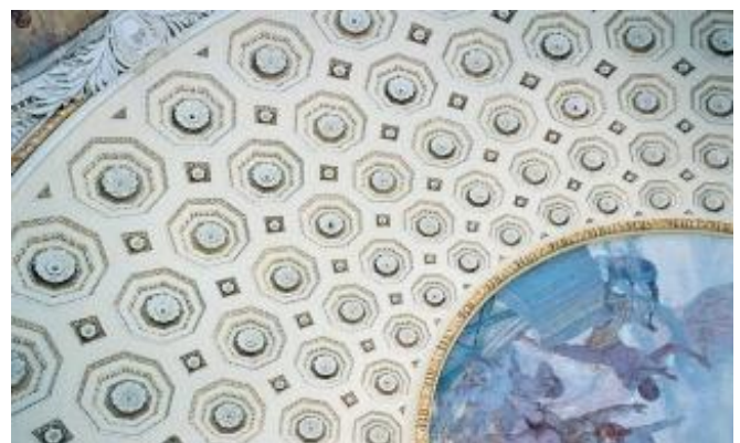
The dome of the US Library of Congress – spot the sprinkler!
