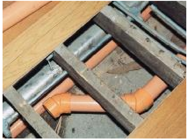
A plastic sprinkler pipe with solvent-welded joints being installed in a convenient ceiling void below the floor joists
