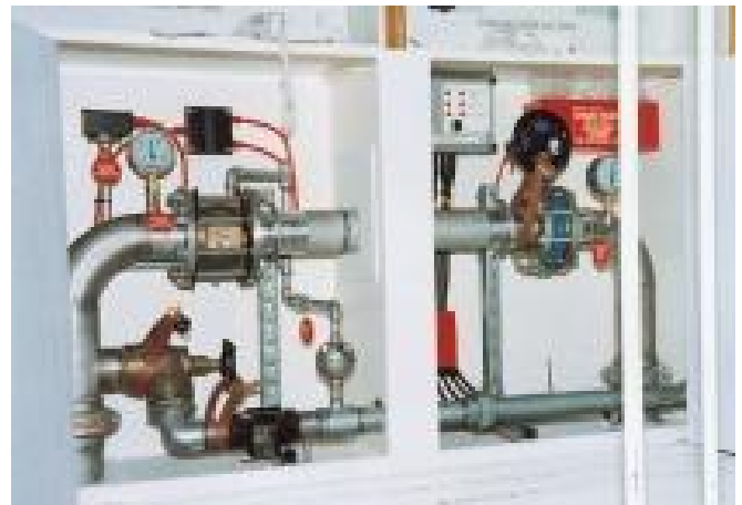
The mechanical works for this sprinkler system are hidden in cupboards beneath two public telephones
