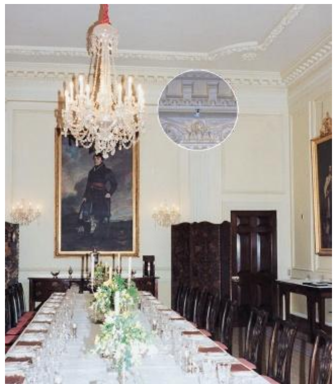
One side-wall sprinkler located above the capital provides protection for this room and its contents. The house remained in continuous use throughout the installation, and by using special dust-extraction drills, this table was laid just one hour after installation.
